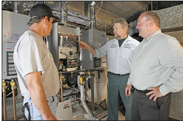
Mike Bauman (right), maintenance director at Steubenville City Schools, inspects one of the three new Rheem tankless water heaters with installer Jim Saltsman (left) and John Vasey, a manager at Rheem distributor Robertson Heating Supply.
