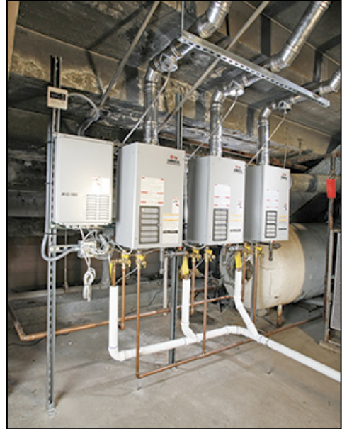
Three Rheem tankless water heaters, shown with their controller (far left), are manifolded together to operate as a single unit. If one heater requires servicing, the other two will continue to feed hot water to the showers in the visitors' locker room.
