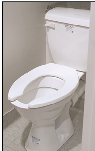
CLOSEUP VIEW OF SANIBEST MODEL INSTALLED IN ONE OF THE SUITES AT BUD WALTON ARENA. THE MACERATING UNIT IS RECESSED BEHIND THE WALL.
