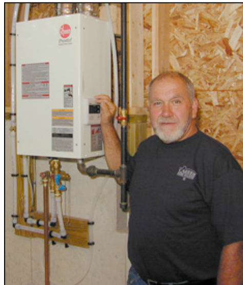
Rejean Carrier of Carrier Home Builders: "I don't have any headaches with tankless water heaters at Chimney Hill, and all the owners are happy with the product."
