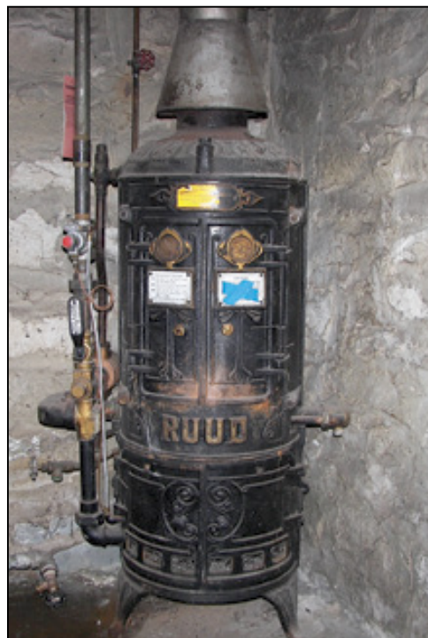
The 1913 Ruud water heater that Jack and Cynthia Vogel discovered – still operating – in the basement of their newly purchased carriage house in Pittsburgh, Pa.
